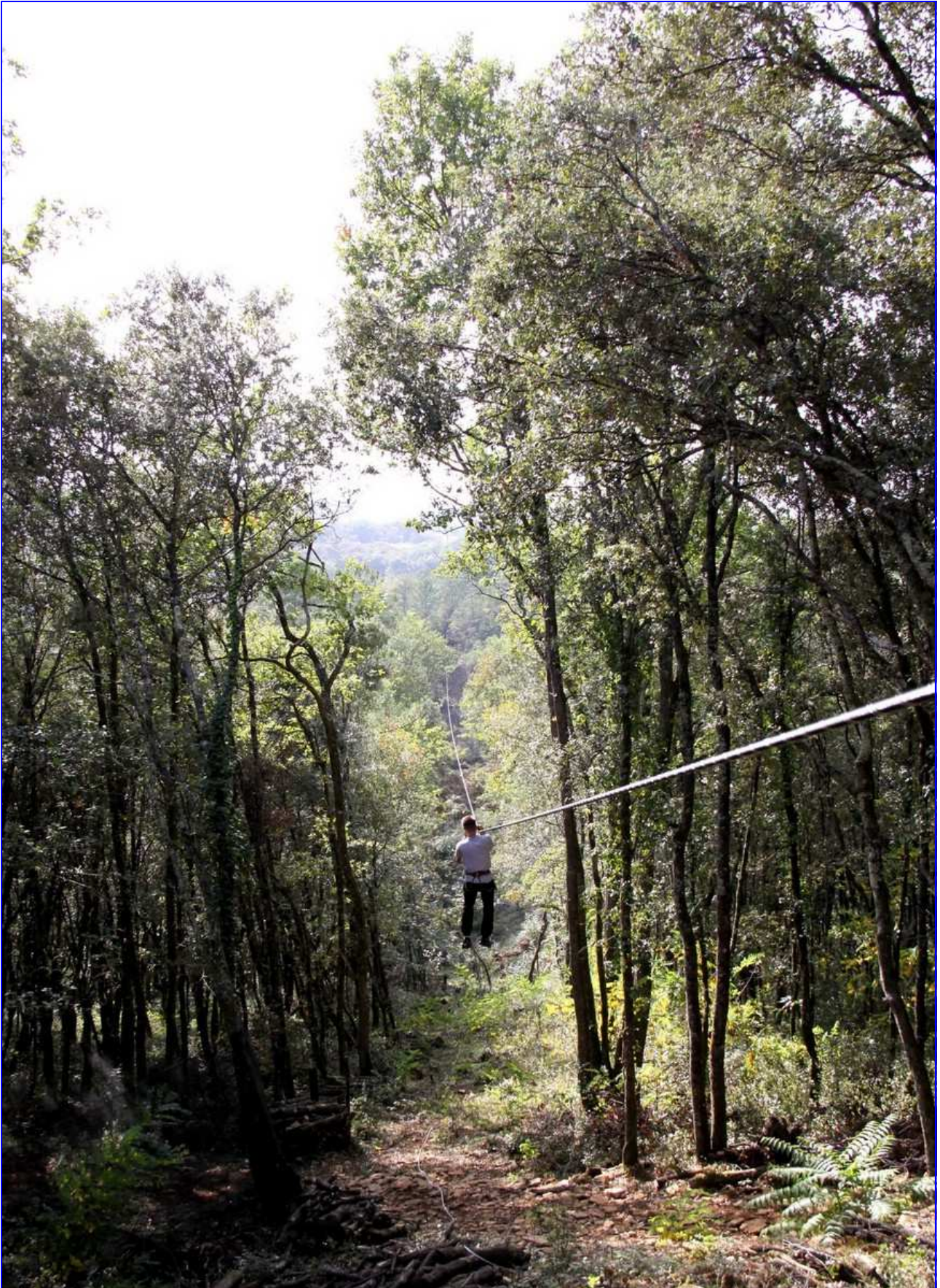
Zip line of 350 metres in Deltex diametre 19 mm. Installation with a very low tension(650 daN) because at this point the slope is very strong (9.4%) and a higher tension leads to a very fast arrival .
